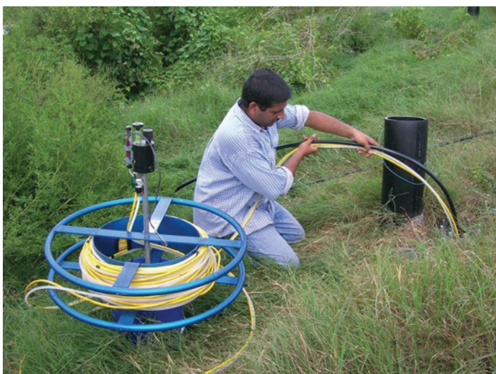
Brajesh Dubey measuring the differential settlement of the leachate recirculation lines inside a municipal solid waste landfill in Florida.
